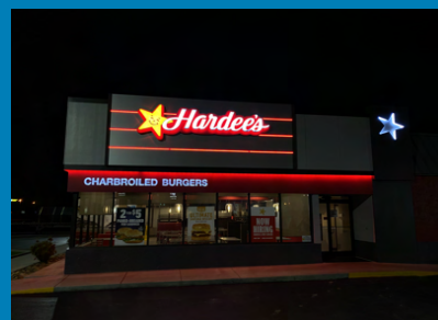
Cove Lighting and LED Retrofits
